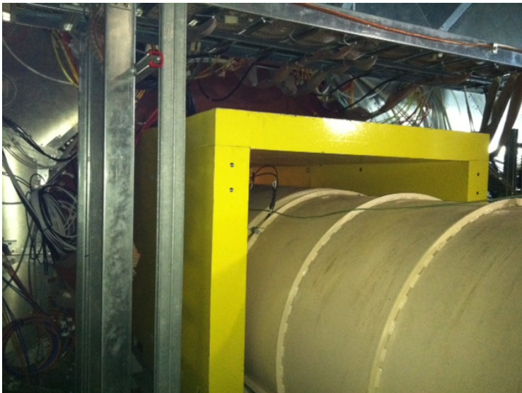
South Tunnel Shielding
